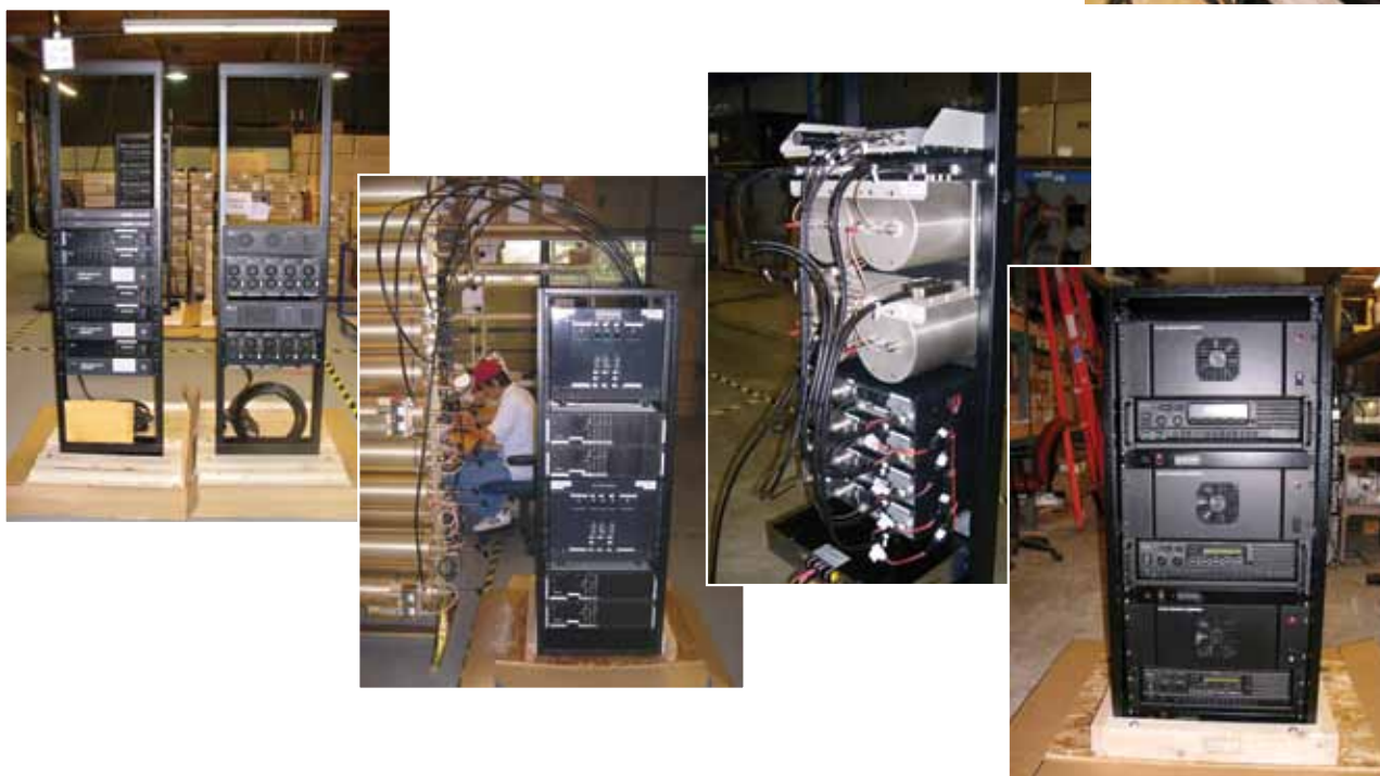
"Real-world" snapshots of various radio systems under construction in the IAS assembly area.
